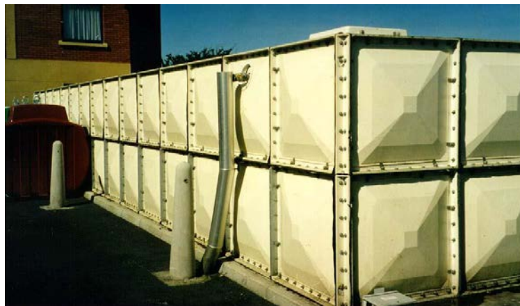
15150 x 4140 x 2000 mm 120,000 litre (26,000 Gallons) Tank Insulated to Format 30. Installed 1998.
